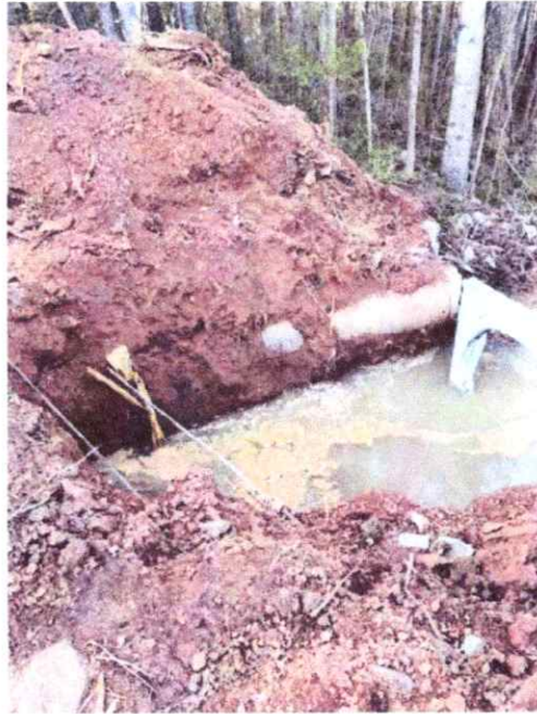
Standing water at the pipe outlet after removal of the first joint of pipe.
